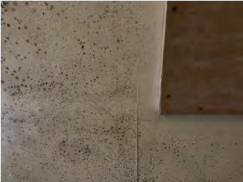
Mold, roof, chinking, exterior wood
